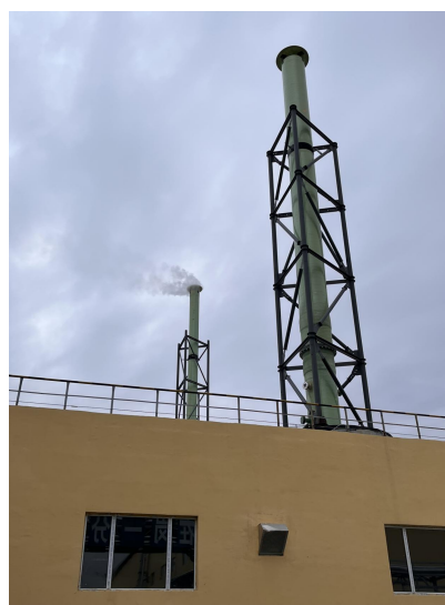
酸性废气和碱性废气排气筒
